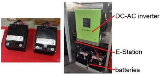
Image 11. Photograph of the buffer batteries and their installation.
